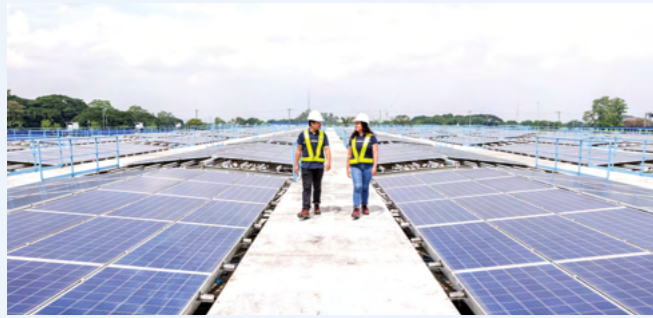
Solar power farms, primarily at the La Mesa Compound in Quezon City, to power water treatment and pumping facilities
